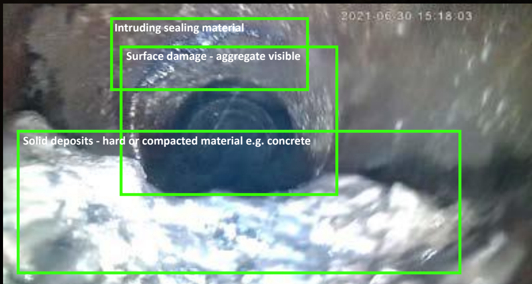
AI AUTOMATIC DETECTED DEFECTS
